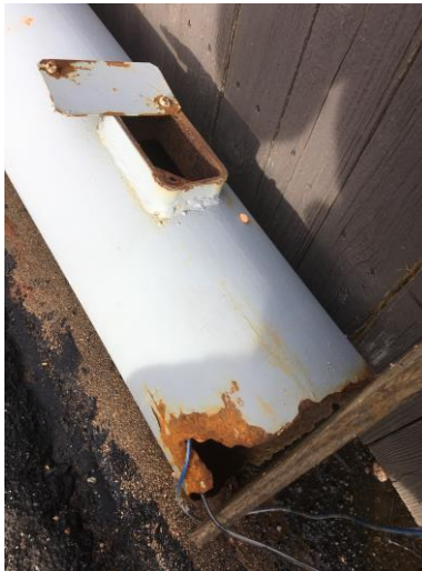
Figure 2: Rusting visible at base of downed pole.
