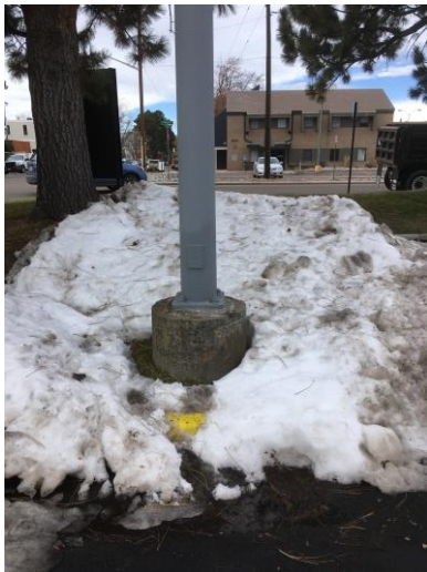
Figure 5: Pole number 7 with large pile of snow plowed around the base.
