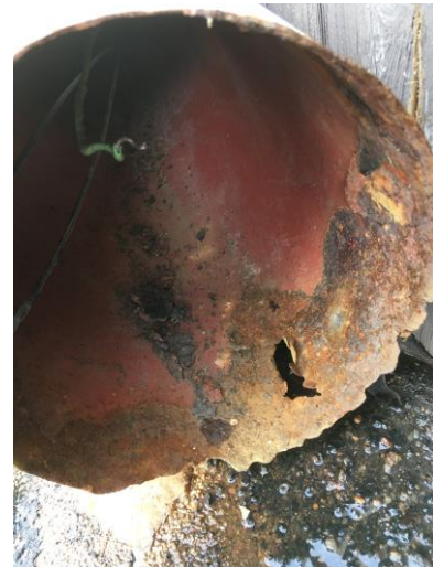
Figure 3: Internal view of rusting at base of downed pole.
